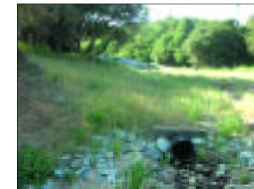
(bottom) Same location following installation of pipe drop and recompaction of soil to fill former gully. Pipe inlet is located behind berm at edge of trees and carries runoff to outlet in foreground. Rock at outlet serves as energy dissipator. The slopes have been seeded with an erosion control mix.
