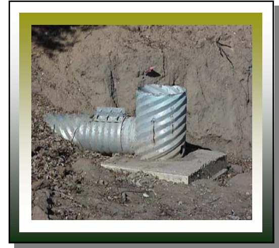
Slotted Riser with six inch base set in concrete.
